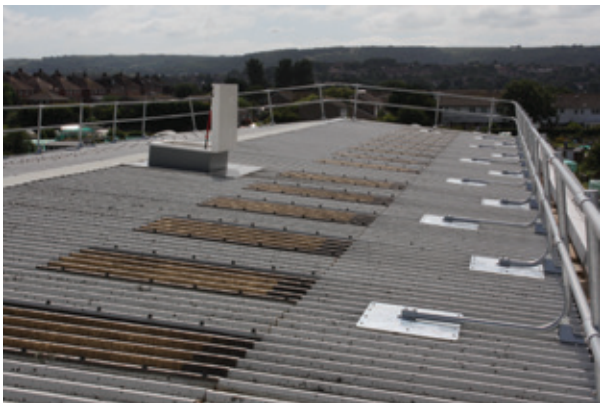
Above Clad Rail System View of installed system.
